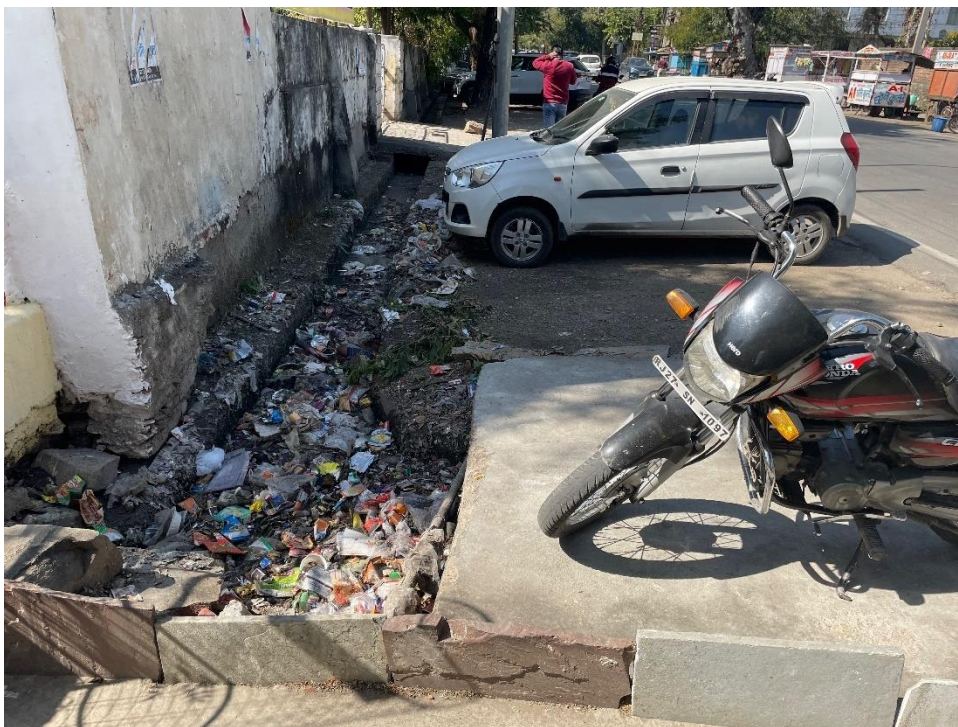
Figure 47: Portion of Storm water drain near Sukhadiya Circle. Source: (Author, 2022)
