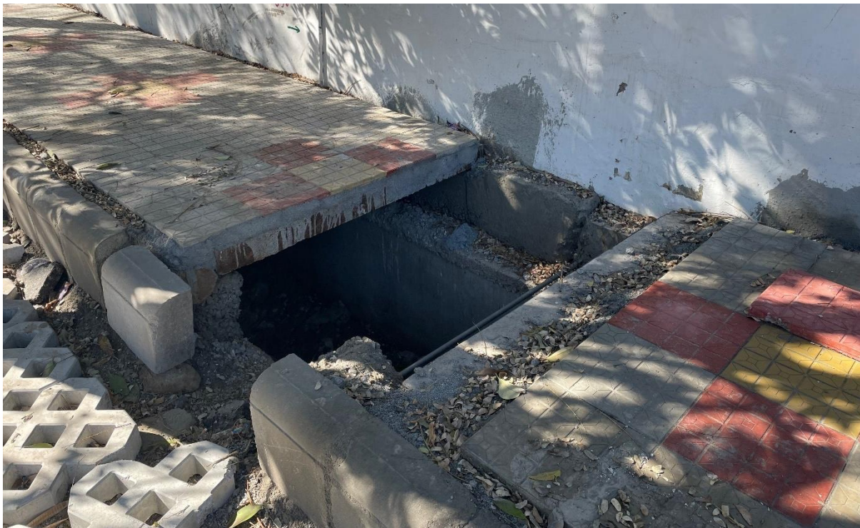
Figure 48: 150mm thk drain cover makes footpath inaccessible. Source: (Author, 2022)
