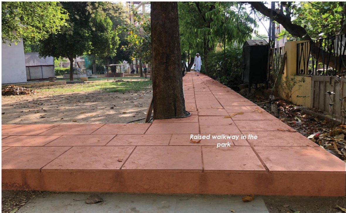
Figure 43 No ramp access for the pathway inside the park
