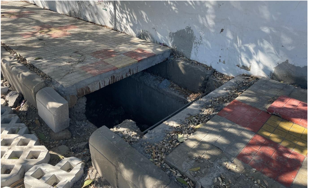
150mm thk drain cover makes footpath inaccessible
